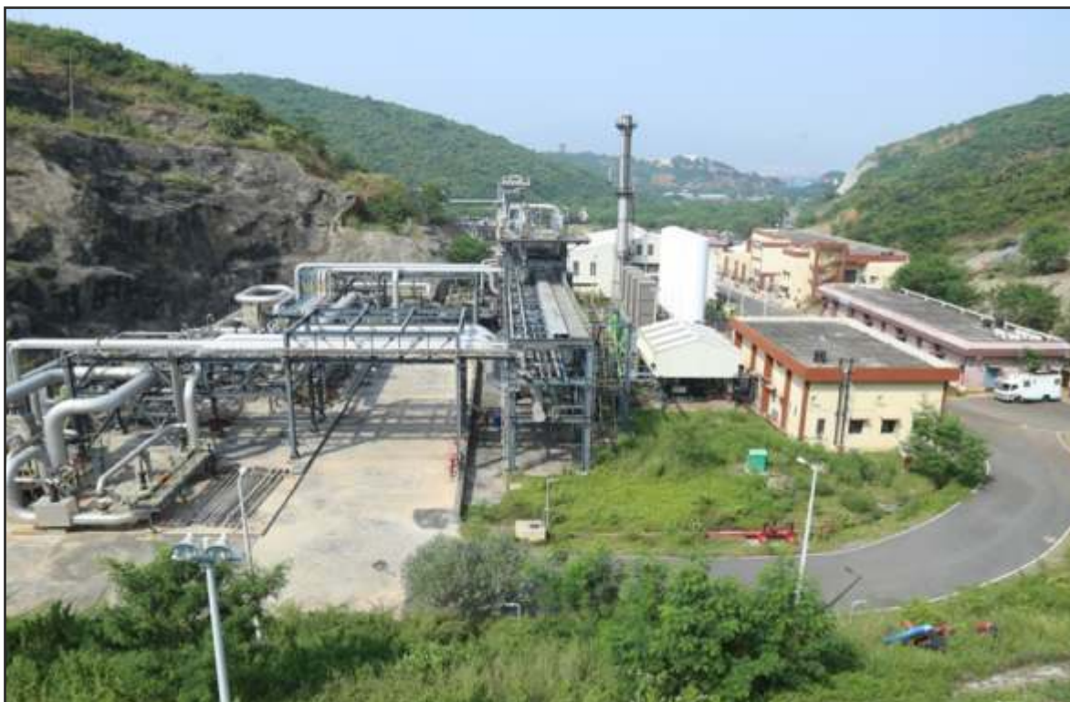
Mangalore (Storage Capacity: 1.5 MMT)
